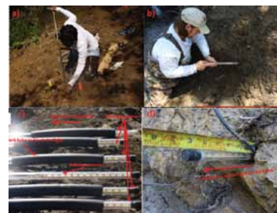
a) and b) Installation Procedure of the PEEPs; c) and d) Calibration of the PEEPs
