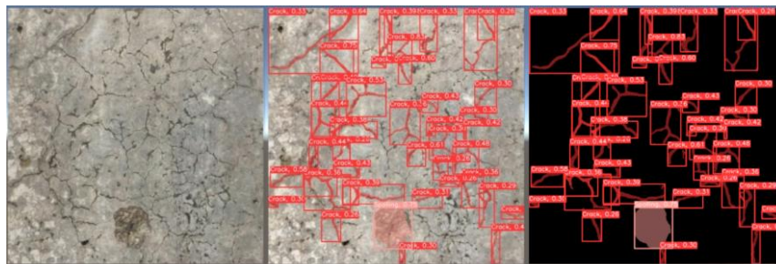
Figure 6. Left – example crack image. Middle – example of output with background image. Right – example of output with only inference mask.
